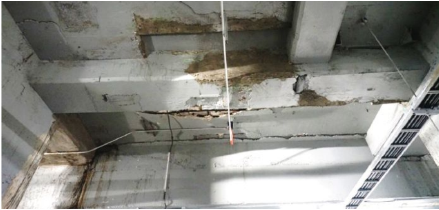
FIGURE 3 Concrete beam exhibiting cracking due to corrosion of rebar and overload.
