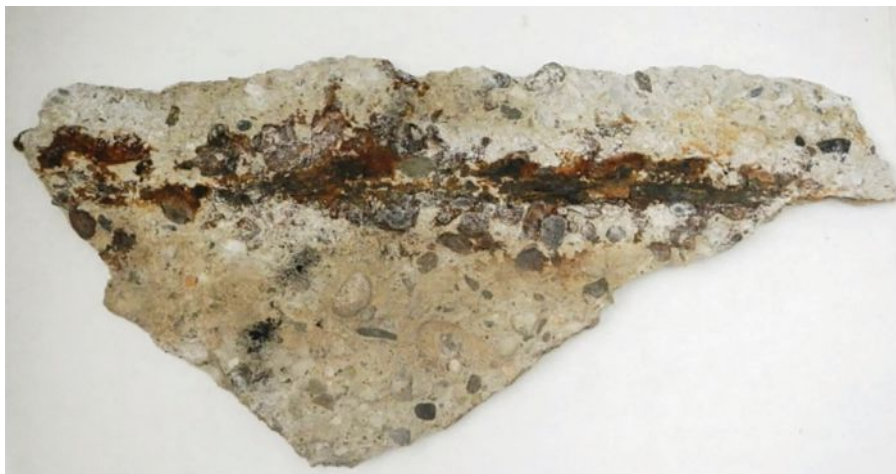
FIGURE 5 Close-up photograph of the rebar inside core sample with thickness loss shown at the top. The corrosion risk was captured early on. Corrosion mitigation and cathodic protection prevented catastrophic failure in a 100-year-old building.
