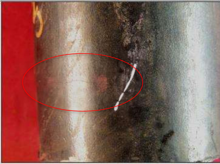
Figure 31: Photograph of the as received failed regeneration heater coil or affected sample which had a crack.
